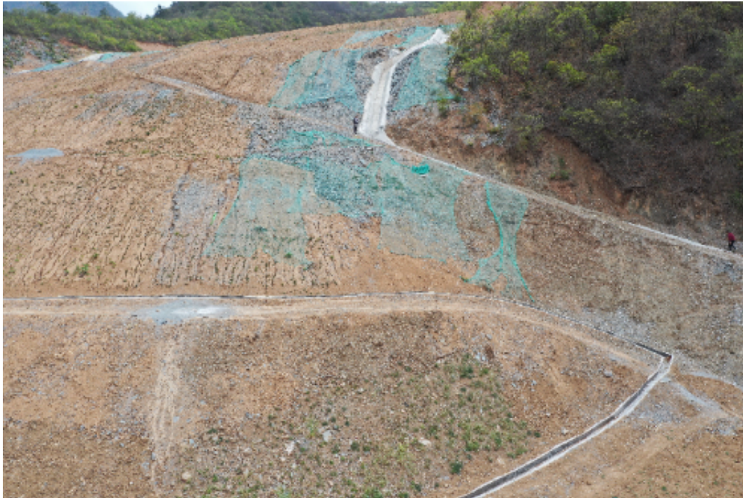
Figure 3 Field photo of rill erosion on the slope of the spoil tips (when there is a clear upslope inflow).
